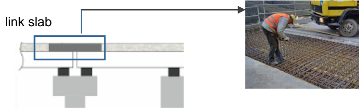
Figure 8: New bridge deck link slab as replacement of joints (scheme and photo)
