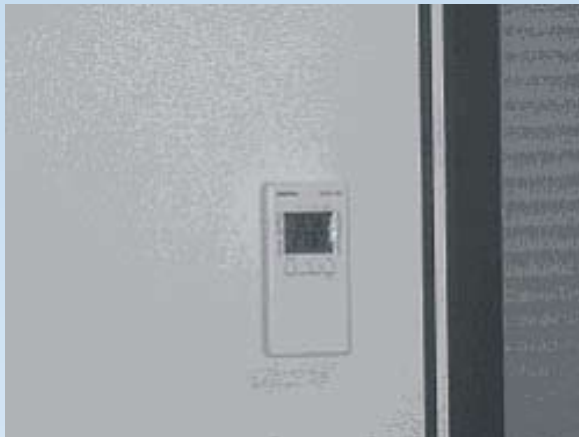
Figure 4. Temperature and CO 2 sensor connected to the BMS.
