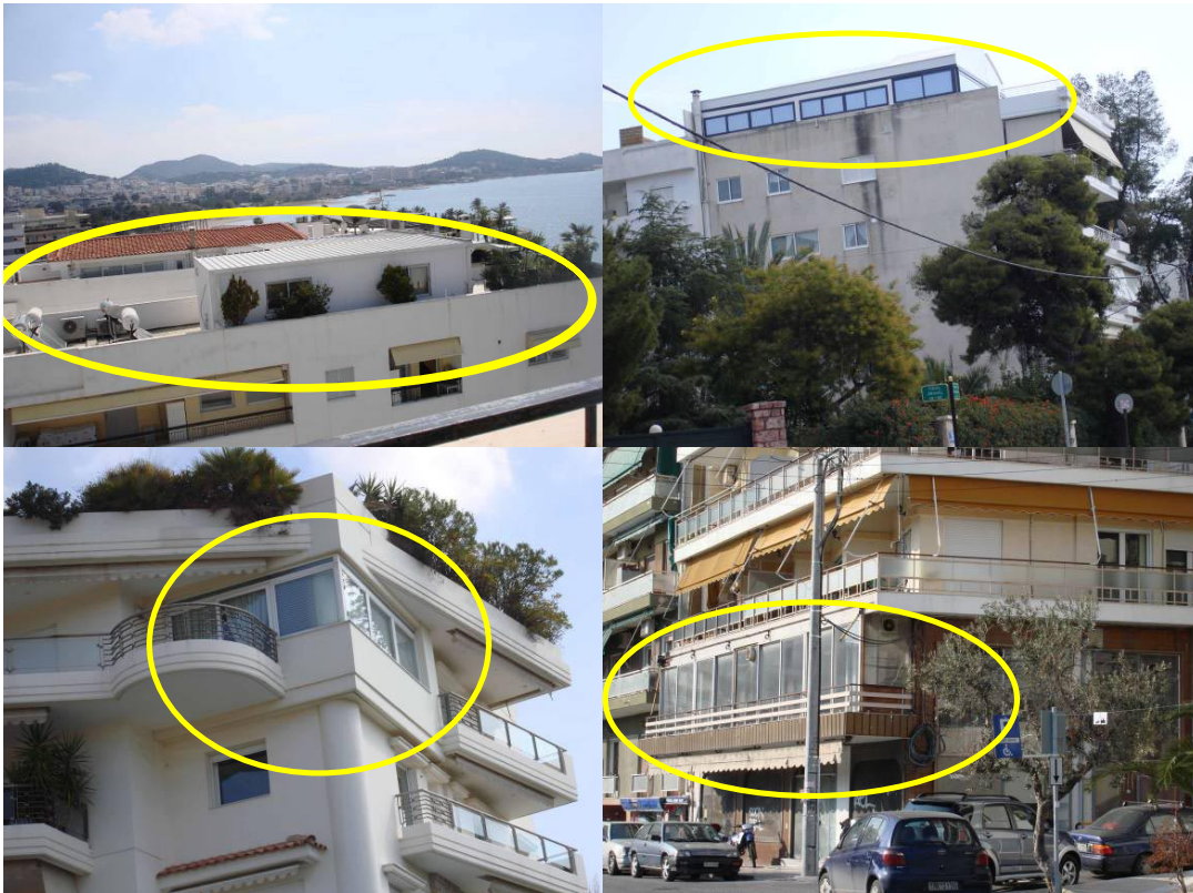
Fig. 8. Illegal construction on top roofs (1 st row) and built up balconies (2 nd row).
