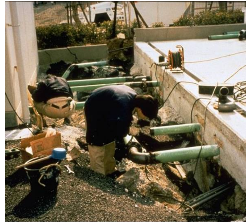
Pipes separated by lateral spreading between a building and adjacent concrete slab near Nakahara Wharf
