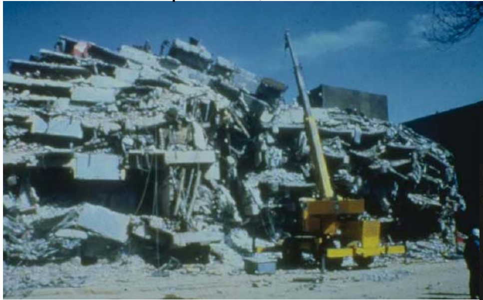
Failure of Top Floors, Hotel Continental
