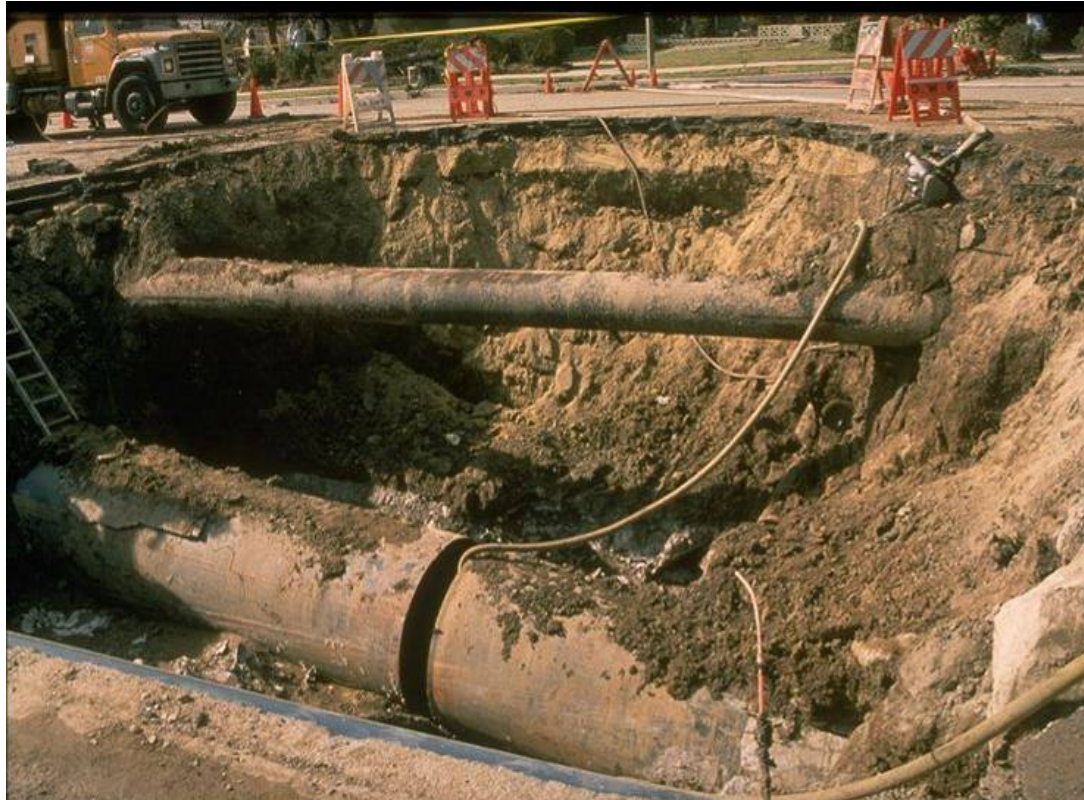
Typical utility pipe ruptured by lateral spreading in Granada Hills on Balboa Blvd
